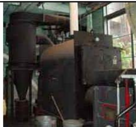
1. 3 MMBtuh Boiler with Gasifier, MA
