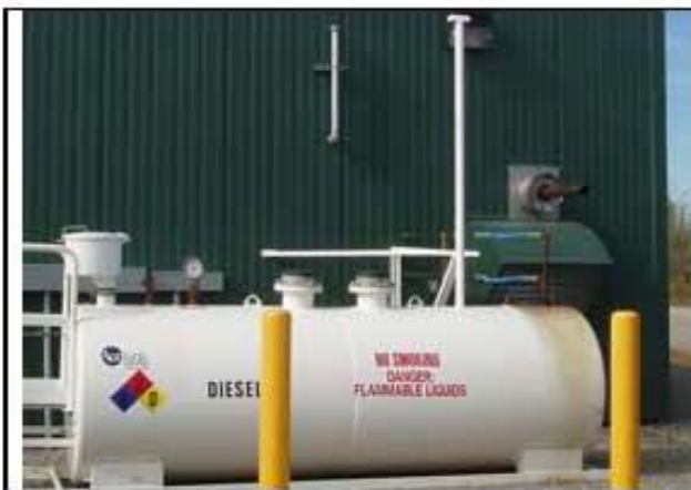
7. Diesel storage, Engine Exhaust
