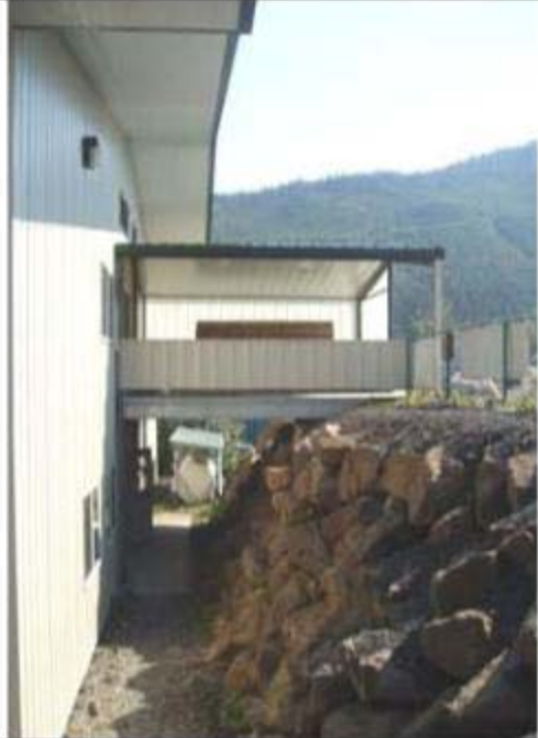
7. Bridge Entry, Fuel Oil Tank Near Boiler
