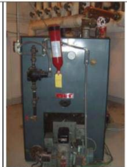
12. Boiler at High School
