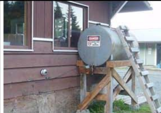
5. VPSO Heater Fuel Tank
