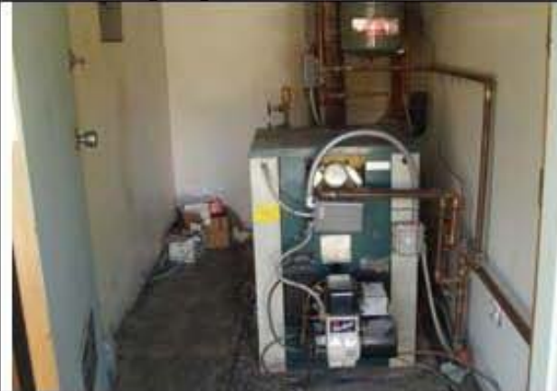
3. City Hall Boiler
