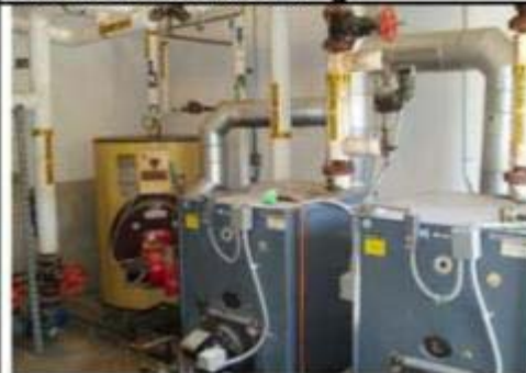
12. Lower Building Water Heater and Boilers
