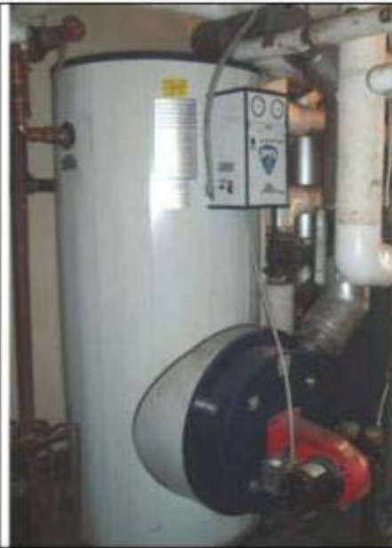
8. Water Heater Upper Building
