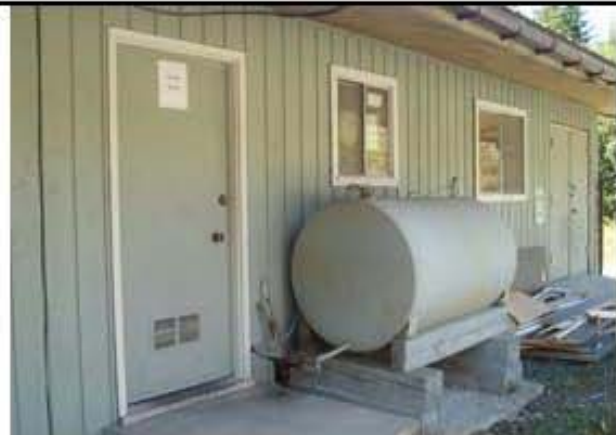
2. Boiler Room and Fuel Tank
