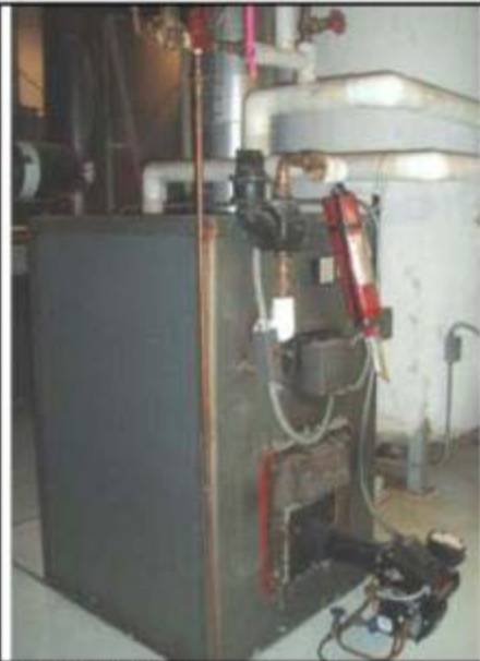
7. Typical Oil Boiler
