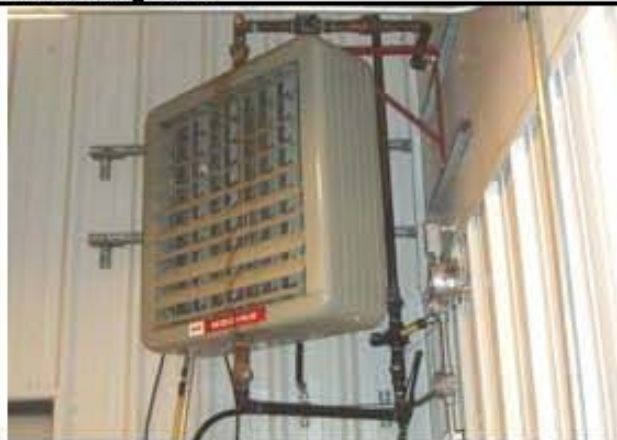
21. Air Heater in Sanitary Plant
