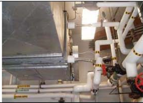
13. Duct Heat Exchanger
