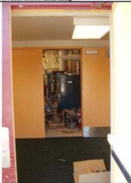
21. New Elementary Boiler Room
