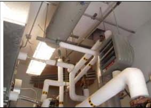
14. Duct Ex changer and Unit Heater
