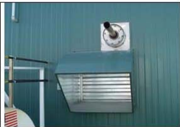
8. Heat Vent and Engine Exhaust
