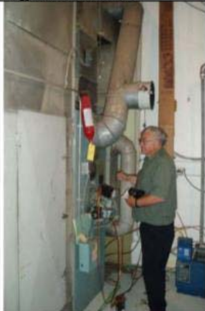
10. Oil fired Air Heater
