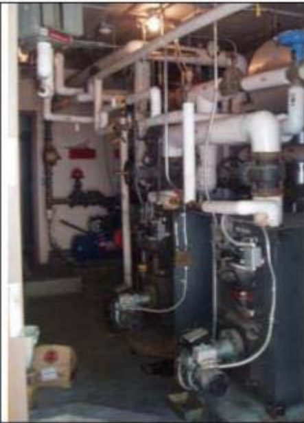
7. Boilers in Upper Building
