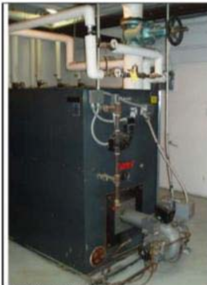
11. Boiler at High School
