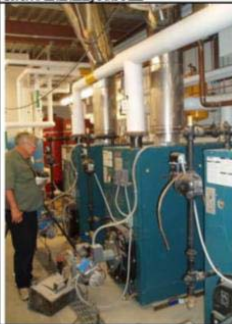
22. 4 MMBtu/h (3 Boilers) + Hot Water
