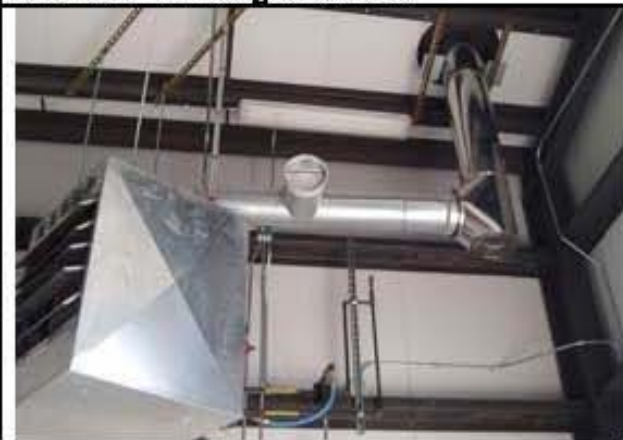
10. Heater and Stack (1 of 2)
