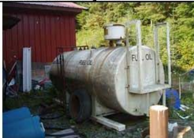
23. Fuel Tank Municipal Waste
