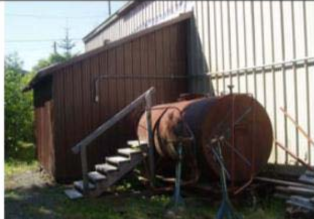
13. Fuel Oil Tank Near Heater
