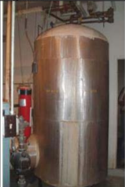
9. Hot Water Heater
