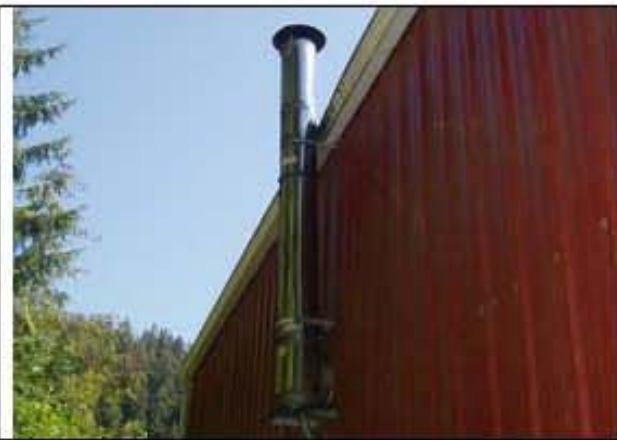
8. Air Heater Exhaust Emergency Services
